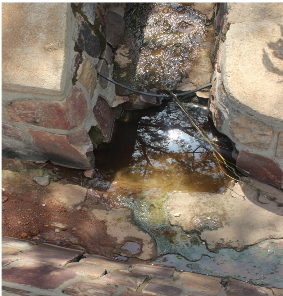
Figure 1: Stagnant wastewater in the drainage channel in KSEZ
