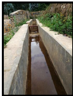
Figure 8: Canal/ Channel at Mudasmwa pico hydro power plant
