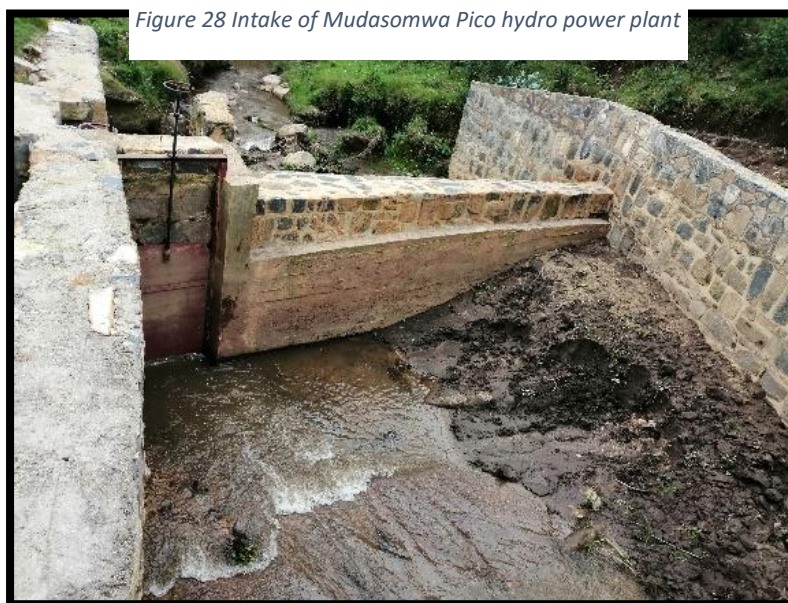
Figure 27: Intake of Mudasomwa pico power plant
