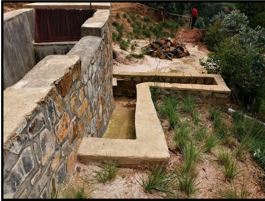
Figure 9: Forebay tank Mudasomwa Pico hydro power plant
