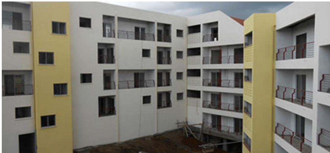
Figure 4.7: Construction site of one of the residential developments labelled as 'affordable apartments'. Source: Agutamba (2015).
