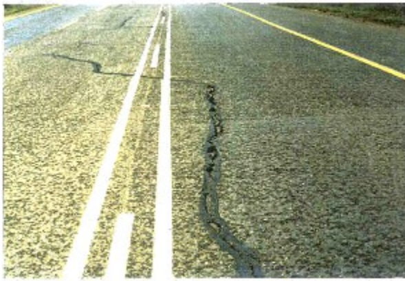
Figure 7: Severe crack degree five
