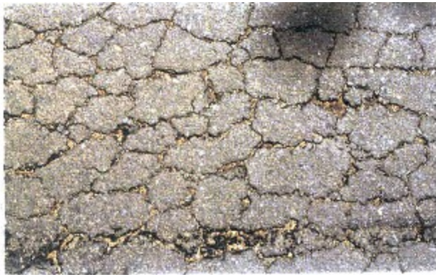
Figure 11: Crocodile cracking degree 5
