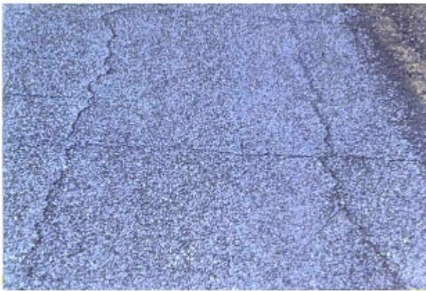
Figure 8: Crack of degree 4 according to TMH9 (2008)
