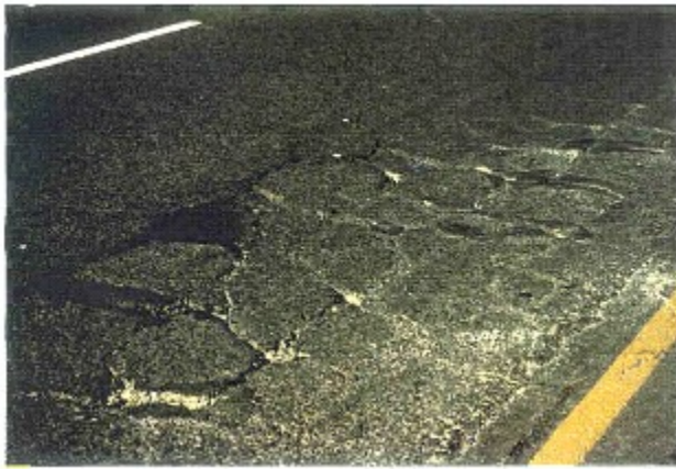
Figure 10: Block crack in severe condition degree 5 according to the rating and extent of the distress (TMH9, 2008).
