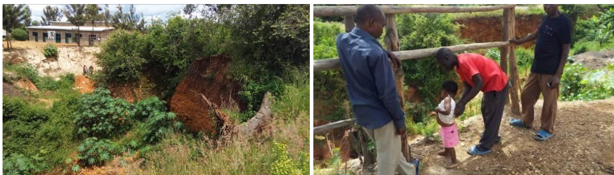
Photo 4-4: Non-fenced, unfilled and abandoned site at H&B
