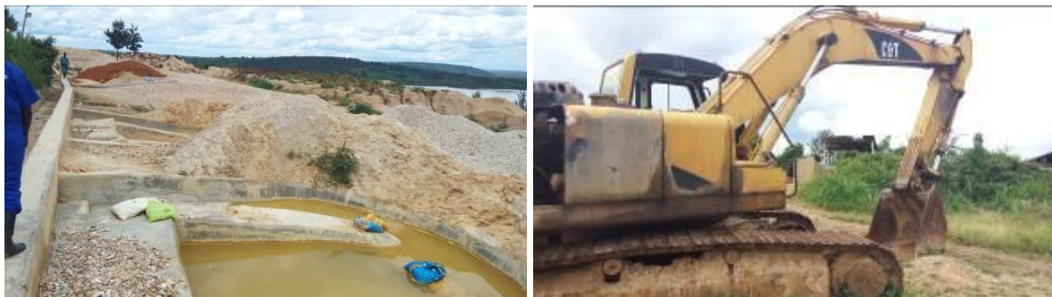
Photo 4-3 Mineral washing facility and an excavator used for various sites clearing activities
