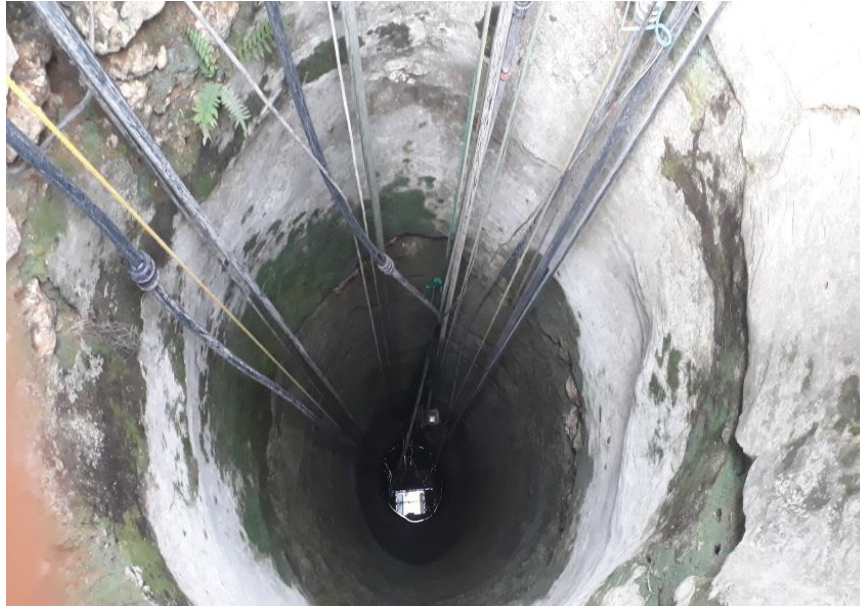
Figure 2.1 Multiple water pumps installed in a community well.
