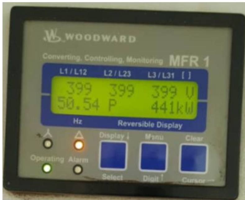
Figure 3: Musarara MHPP generator production display unit.
