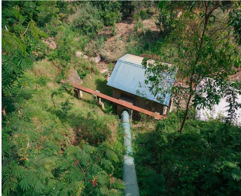
Figure 2: Penstock of Musarara mini-hydropower plant with 60m of head.
