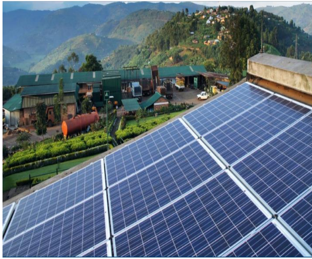
Figure 2. 50 kWp Installation at SORWATHE
