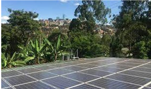
Figure 3.20 kWp Installation at KIGALI GENOCIDE MEMORIAL
