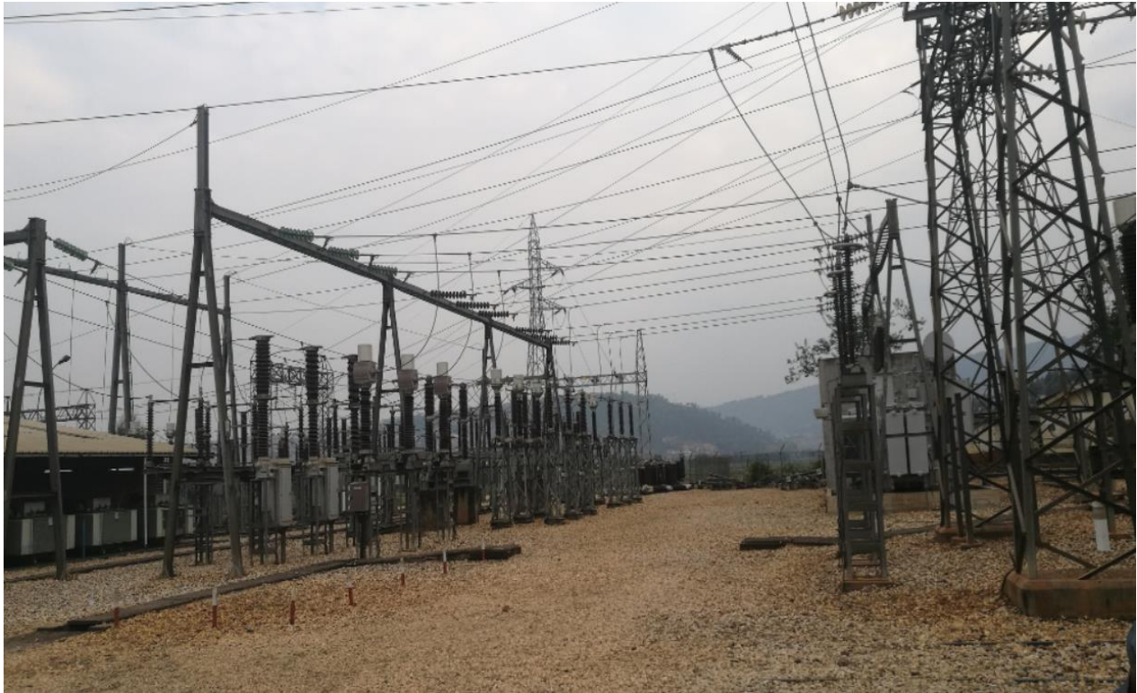
Figure 3. 2: Photo Image for Jabana Substation
