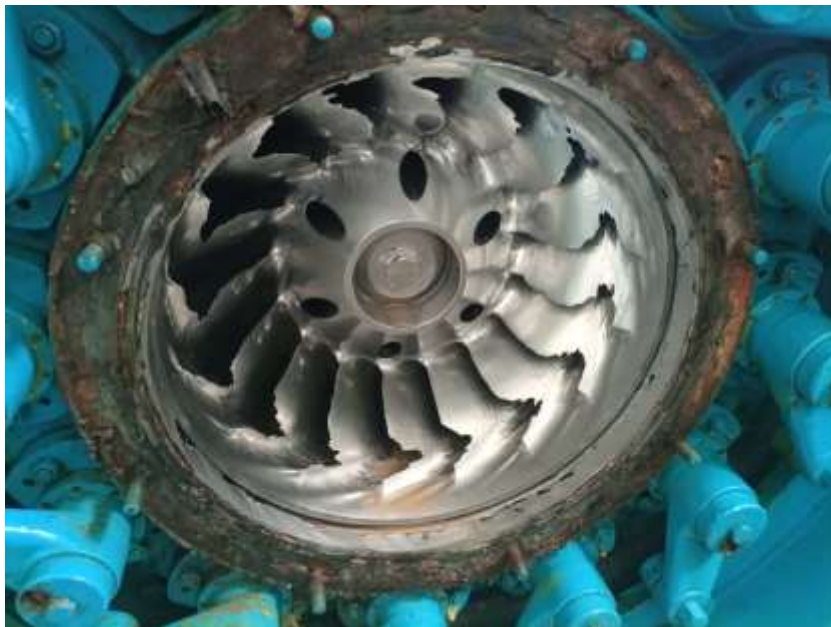
Picture 4.3 Combined effect of sediment erosion and cavitation to runner status
