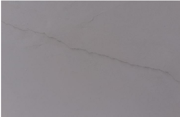
Figure 22: Cracking in the Gatuna walls
