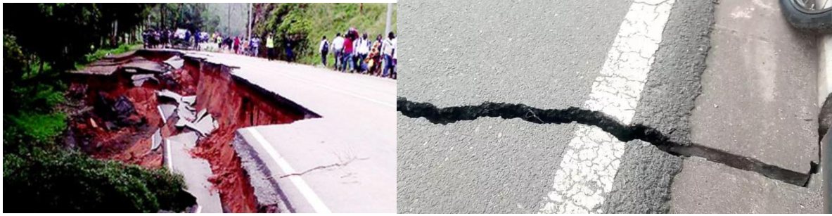
Figure 1: Deep crack caused by heavy rain in road of Kigali-Musanze, at Gakenke, Source: Newtimes, 2013), left and road crack in Rubavu, 2021(right, Newtimes, 2021).
