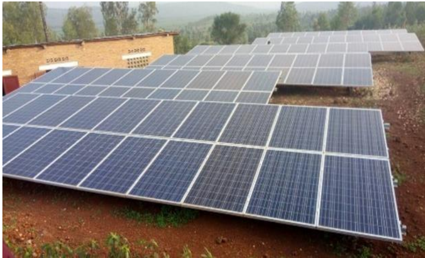
Figure 2 : NESELTECK Located in Kirehe District with a capacity to generate 30KW
