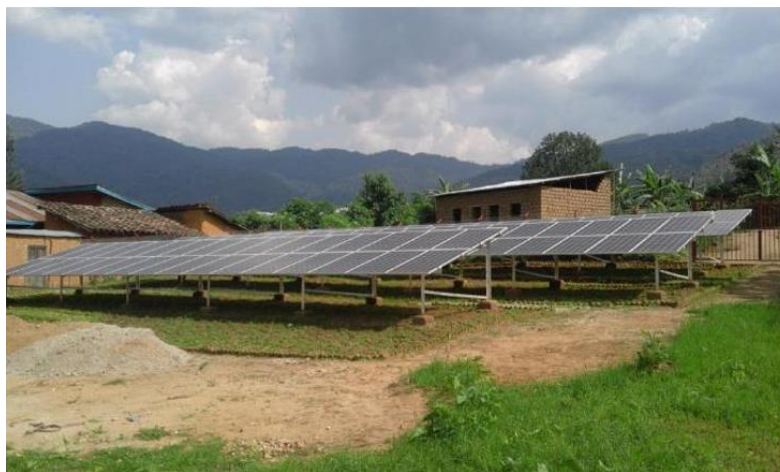
Figure 3: RENERG located in Nyamasheke District with a capacity to generate 30KW
