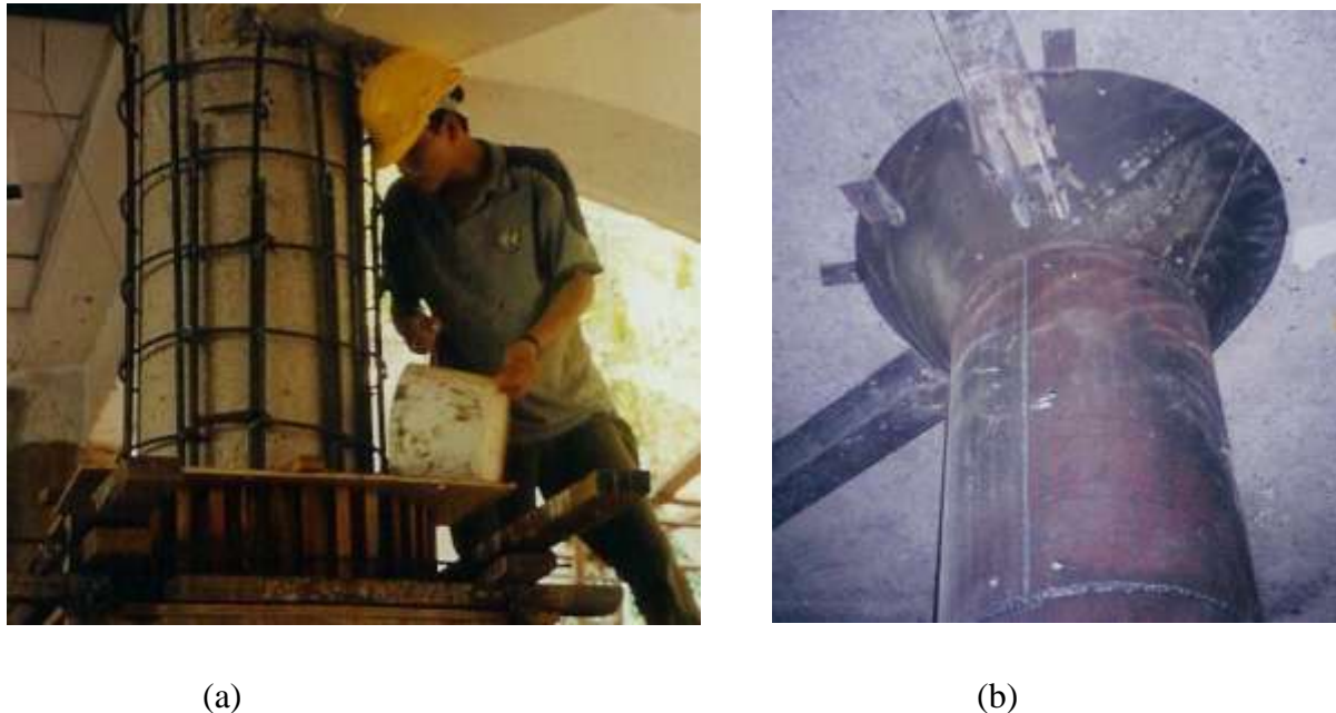
Figure 2.2: Traditional methods of strengthening: (a) concrete jacket, (b) steel plate bonding. (Y. Chhabra, 2013).
