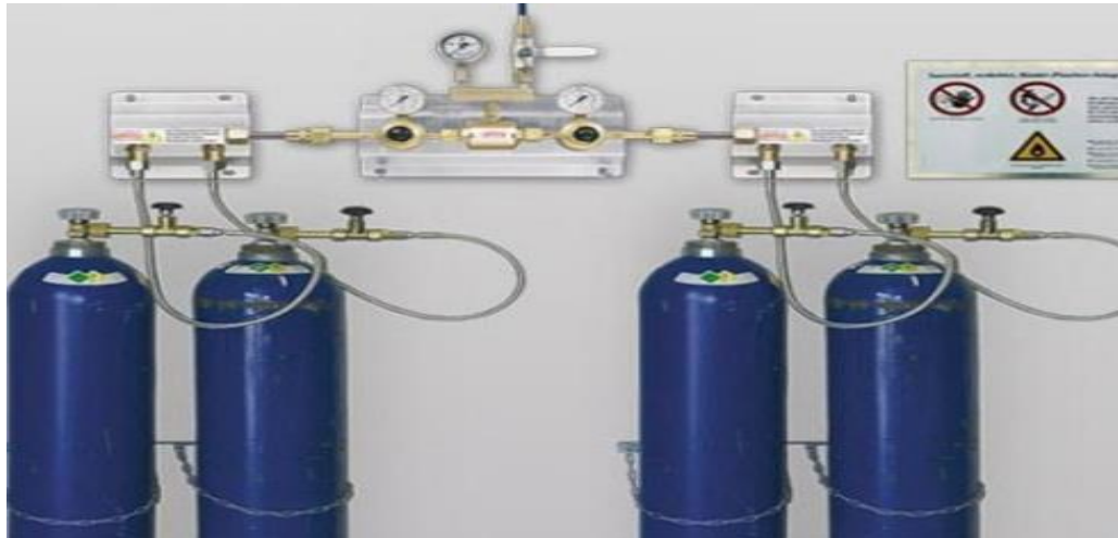
Figure 3.6: Central Oxygen supply Manifold
