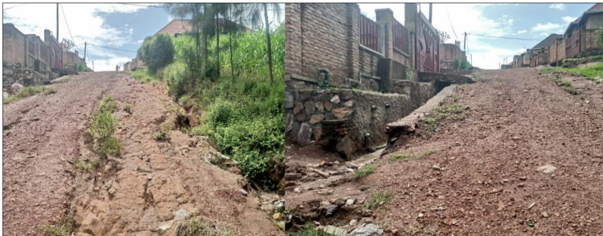
Figure 19:Gullies resulting from the rain water
