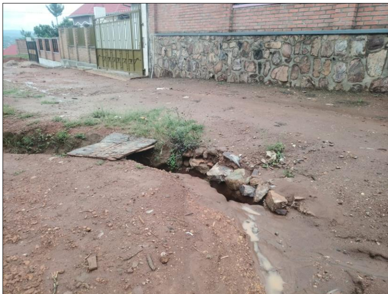
Figure 21: Gullies deteriorating Roads within the study area
