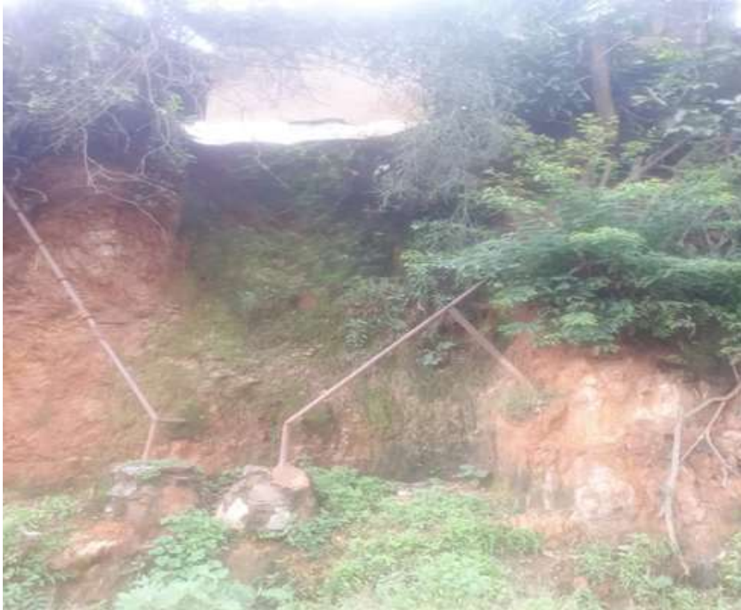
Figure 23: Impact of landslides on the existing infrastructures in study area / Nzove cell (Source: Author)
