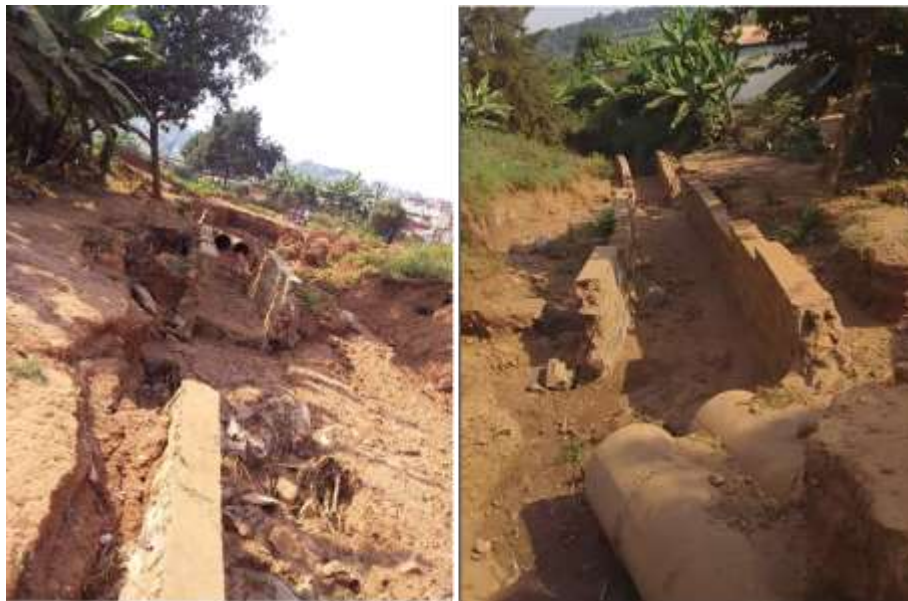
Figure 19.c: Culverts are INADEQUATE to handle storm water in Bisambu-Bigo ravine
