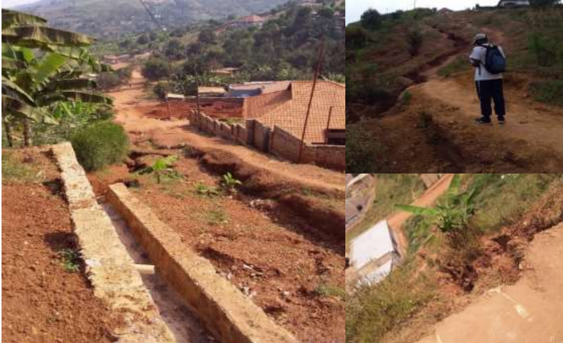
Figure 20.c: The changes in storm water flow direction have led to erosion and road damage
