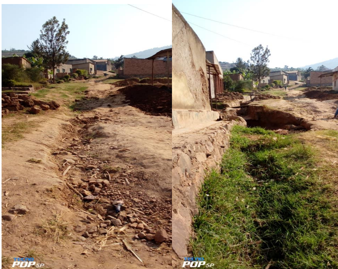
Figure 9: Road degradation in Rutonde
