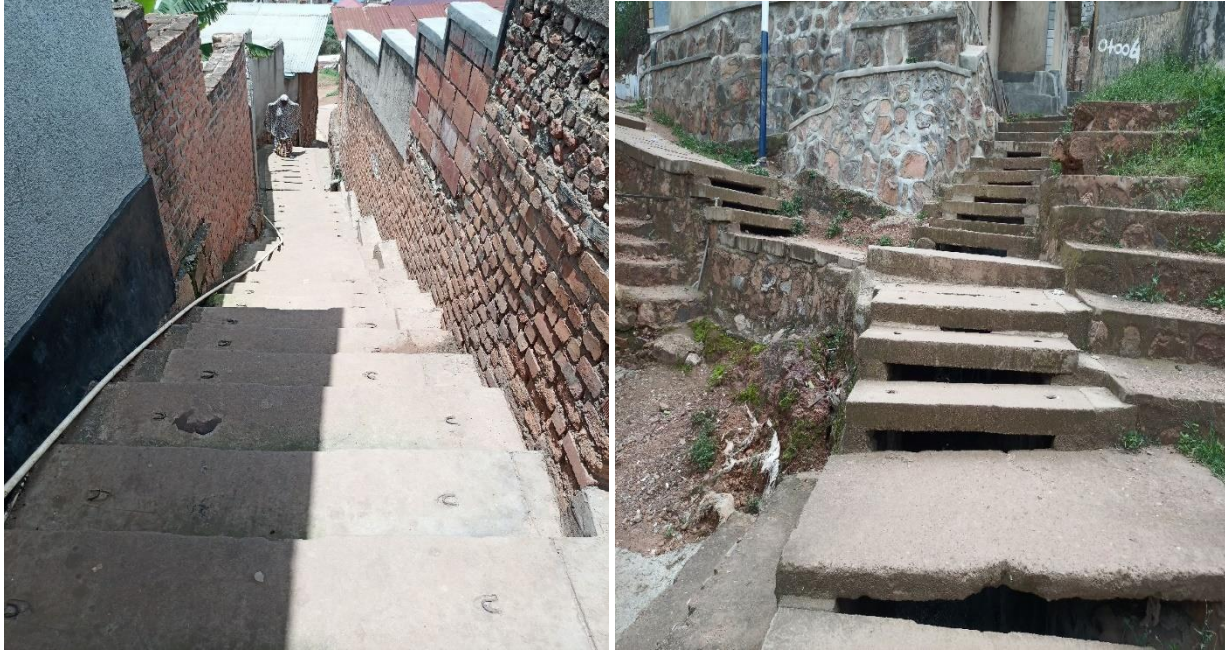
Figure 10. Footpaths serve as small drains (Source: Field survey)
