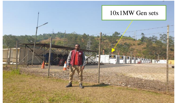
Figure 3: 10 x 1MW oil-fired plant operated by IPP “So-Energy Ltd” at Mukungwa 1 HPP
