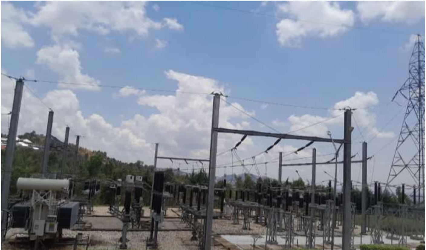
Figure 9: Photo Image for Kigoma Substation
