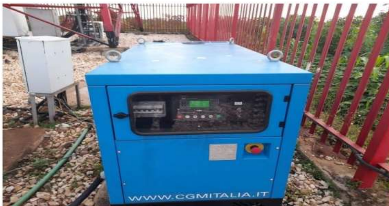
Figure1: Kayumbu base station site's typical diesel power generating system.
