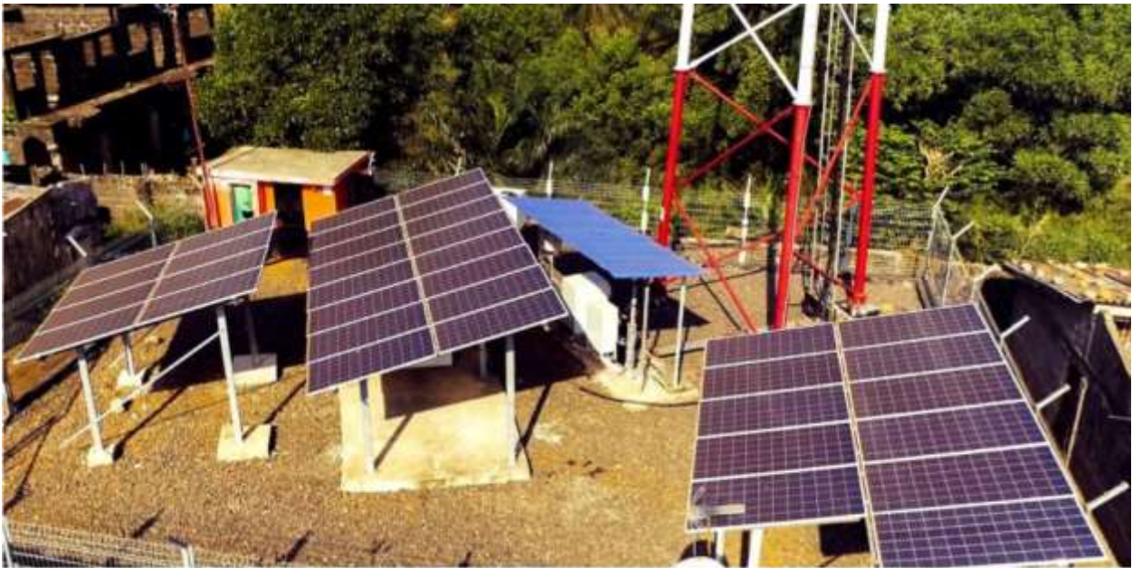
Figure 6: Telecom tower powered by solar PV energy.
