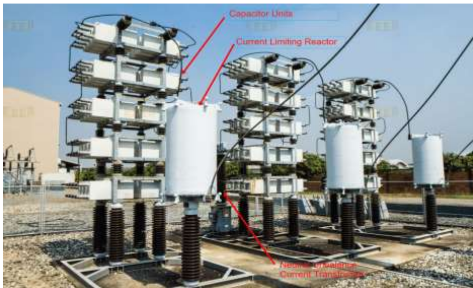
Figure 3 Reactive Power Compensation Capacitor banks[9]
