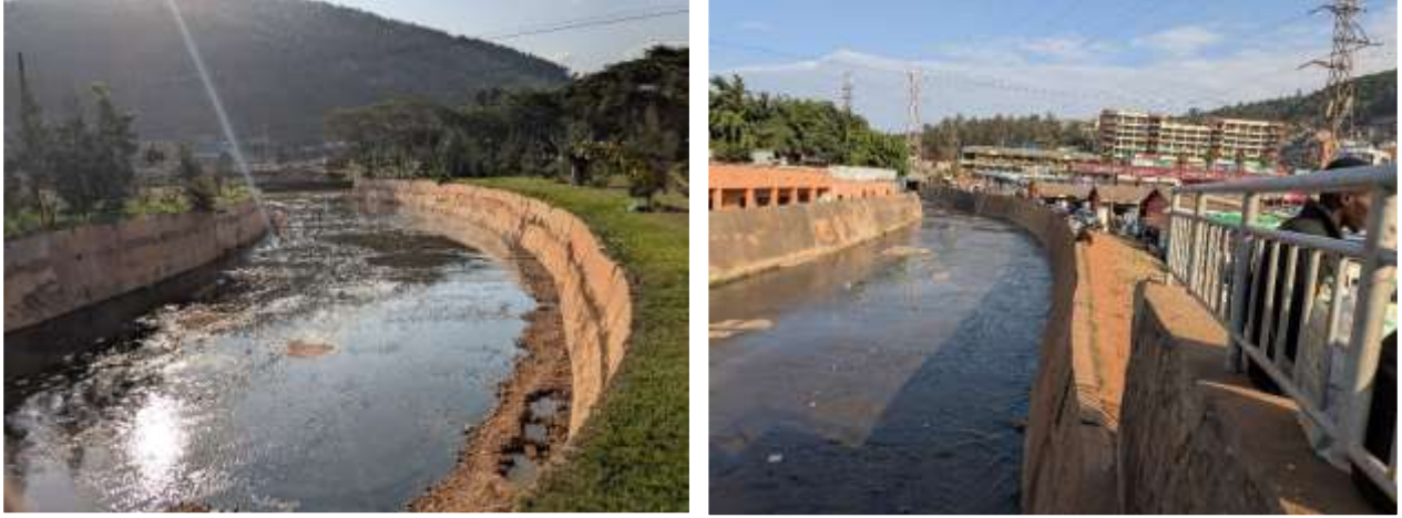
Figure 9: Left: Picture over Mpazi drainage. Right: View of the Mpazi Drainage facing northwest. In the distance, the confluence with the Nyabarongo River and the National Road 3 bridge can be seen.
