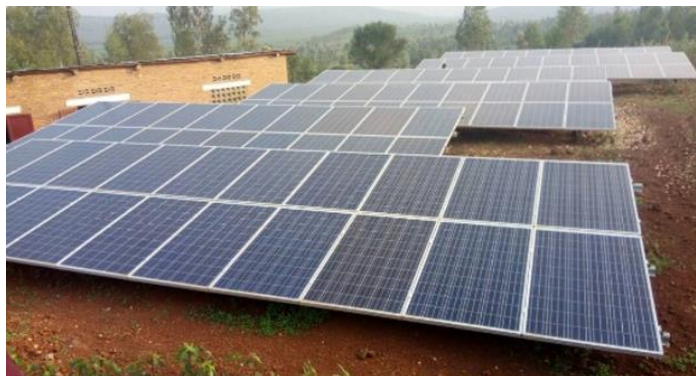
Figure 8: Rushonga 30kW AC Mini-grid constructed in Kirehe District[8]
