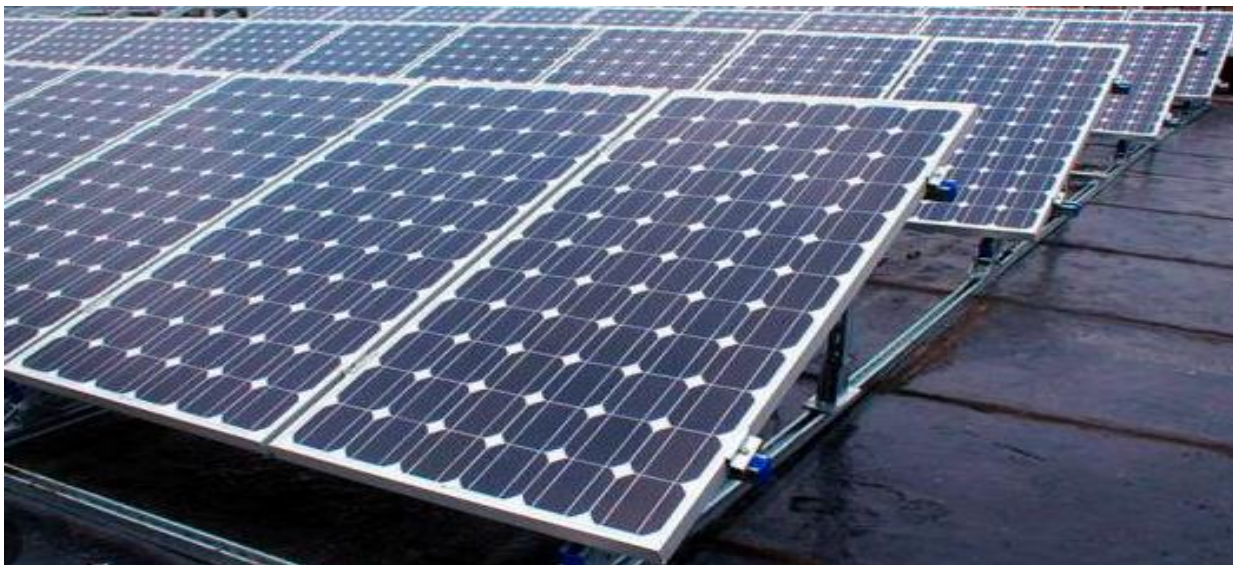
Figure 2.2: Fixed Solar system
