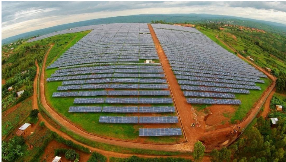
Figure4.1. Rwamagana solar power plant [45]
