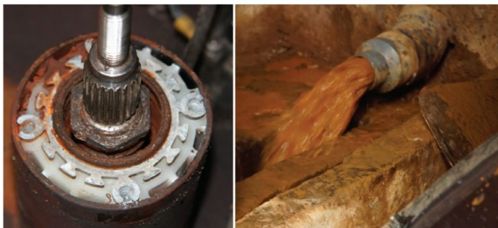
Fig. 2. Damaged parts and water quality. Left: Damaged bearing and housing. The bearing is completely missing (rusted opening below the thrust nut). Right: Water quality when cleaning the turbine inlet. Although the water got clearer after a while, silt concentration is typical of most streams in Rwanda.
