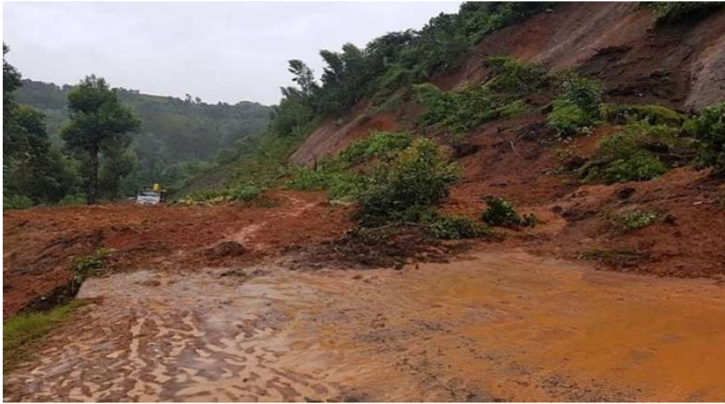
Figure 1- 3 The Failure of a road in Rwanda western/Province Rutsiro District
