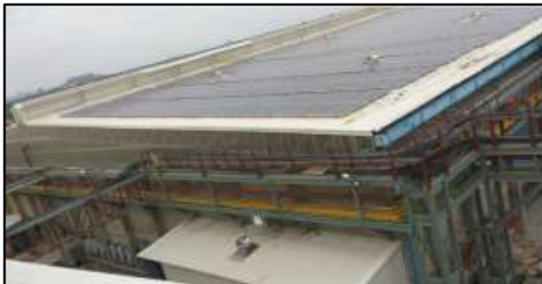
(e) Flush mounted solar PV
