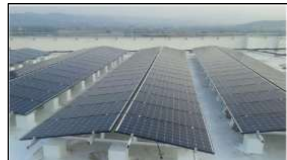
(h) East-west mounting of solar modules
